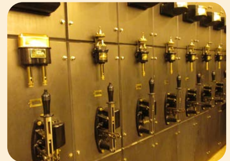
A switch panel occupied a bank of meters, but no one got near them. The switches might not have been live? Maybe?
